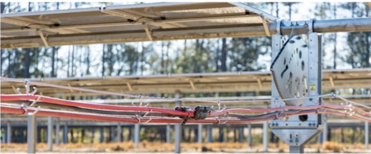
CMS (Cable Management System)
