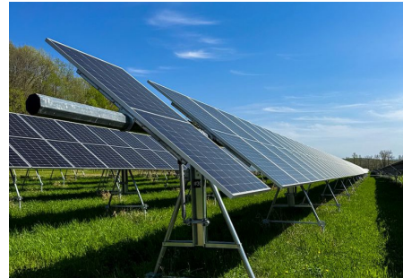
3.3 MW, A-Frame Middlebury, VT
