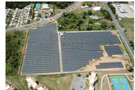
3.7 MW, Ready Rack Fajardo, Puerto Rico
