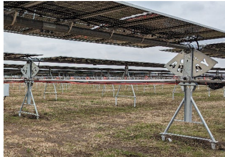
19.5 MW, A-Frame Clark County, IL
